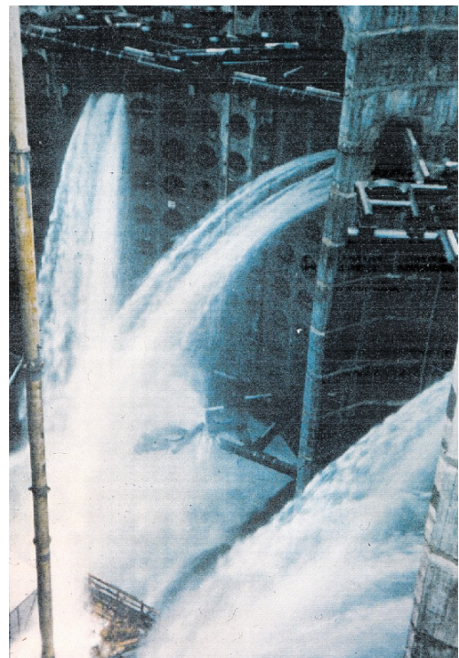
Figure 5.8 Leaks through the External Wall during the Installation of CDP1
